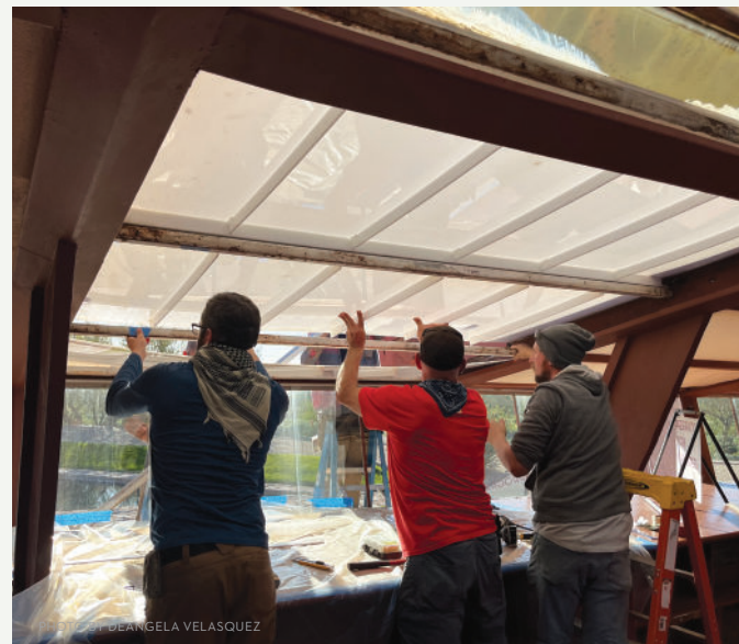
PRESERVATION TECHNICIANS DISASSEMBLING ACRYLIC ROOF PANELS IN DRAFTING STUDIO, FOREGROUND: JUSTIN DAVIS, KELLY HOAGLAND, CHRIS HALMI. BACKGROUND: AKIM MIMOUN, MICHAEL LUST. 2025.
