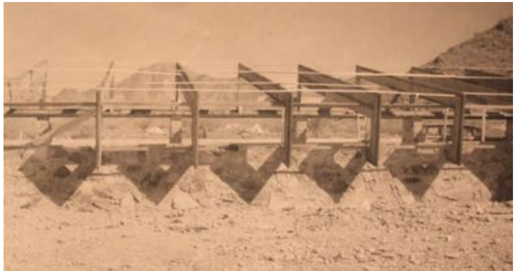
Figure 8-8 - Construction of the Drafting Studio, ca. 1939 (The Frank Lloyd Wright Foundation Archives, The Museum of Modern Art | Avery Architectural & Fine Arts Library, Columbia University, New York).
